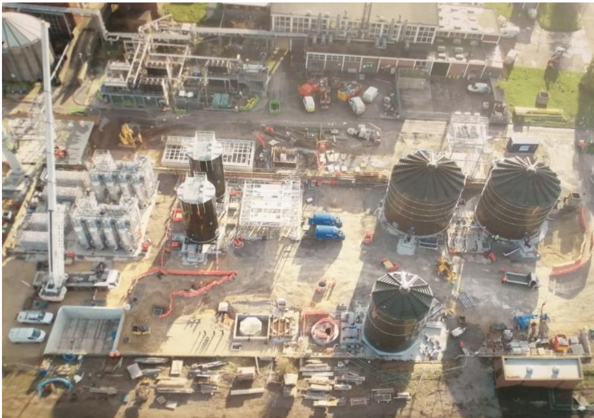
Site aerial view – prior to any install of the odour control package
